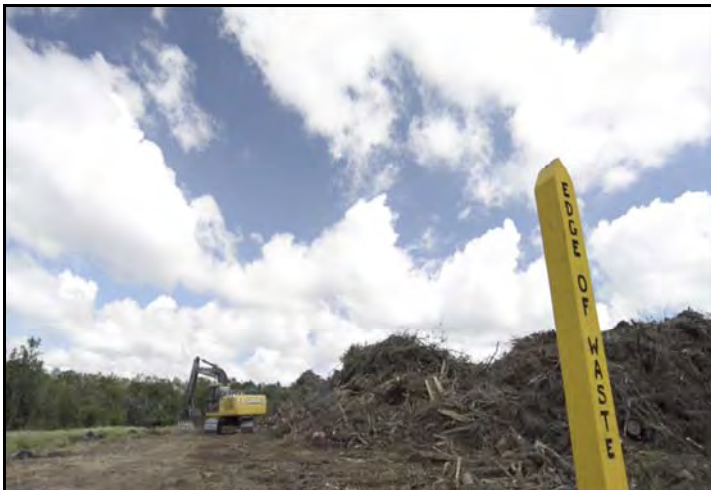
Apalachee Parkway Solid Waste Management Facility
