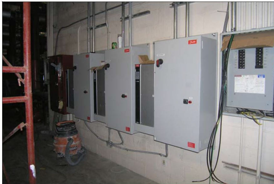
Architectural & Engineering Services- Electrical Panels
