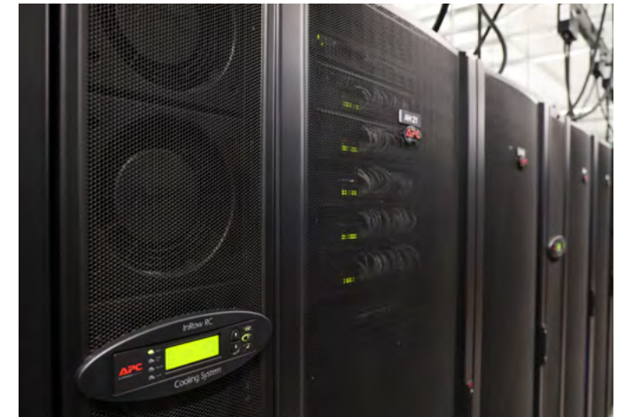
Public Safety Complex server room
