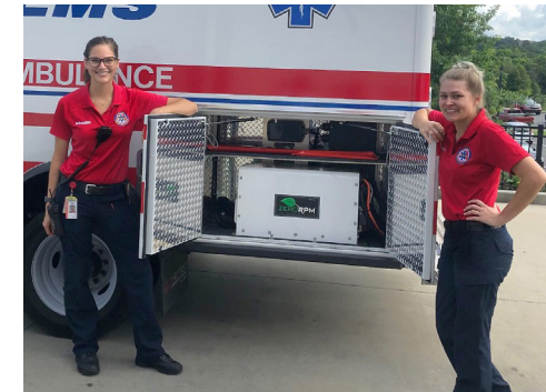
On-board battery systems installed on EMS ambulances
