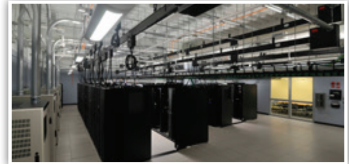
Public Safety Complex Data Center
