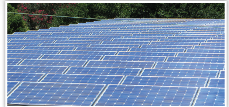
Solar Panels at Net-Zero Facility
