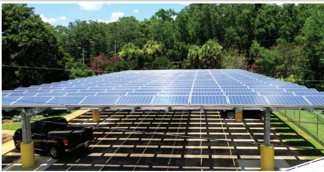
Leon County Cooperative Extension Net-Zero Facility
